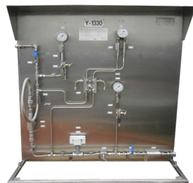
Produced water, sand and solid sampling panel
