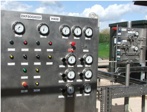
Single Wellhead Control Panel
